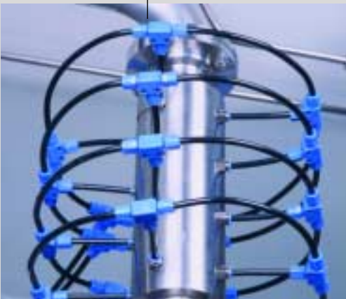
Oxygen mixing pipes.
