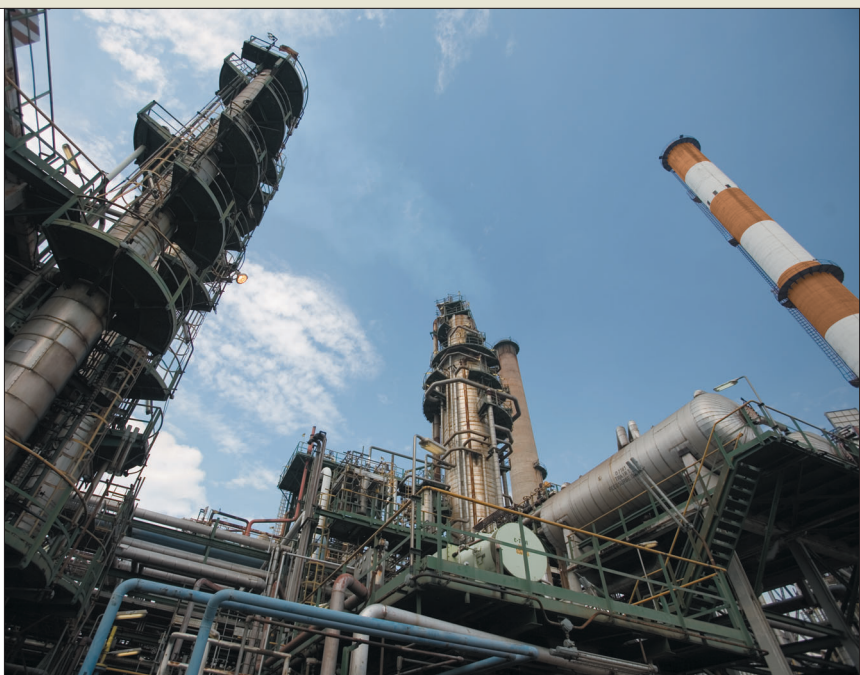
ExxonMobil's Singapore Refinery Visbreaker was recommissioned in 2005 – one example of how we are increasing refinery conversion and overall refinery capacity utilization.
