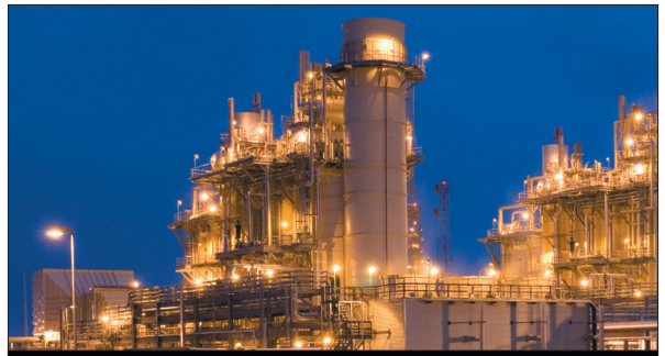
In 2005, ExxonMobil commissioned two of these 160-megawatt cogeneration trains at Beaumont, Texas. Cogeneration is up to twice as efficient as traditional power generation technology.
