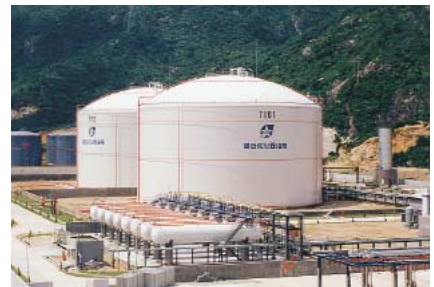
Refrigerated LPG import terminal in Shenzhen, China
