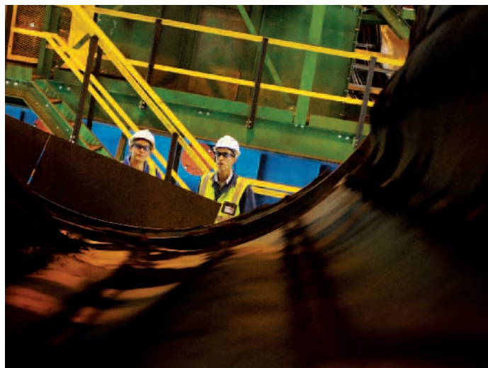
The Bokamoso pelletising project at Wonderkop in South Africa reached full production capacity during 2008, exceeding name-plate capacity by more than 15% for three consecutive months
