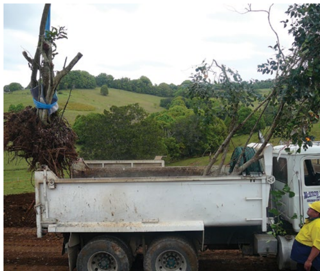
Figure 6.6 Lowering Macadamia tetraphylla transplant into truck for transport to recipient site after excavation and pruning. Ballina Bypass translocation project. (Photo: A Benwell)
