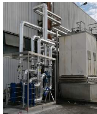
Fatal energy re-use at our Pont-de-Roide unit (heat pumps).
