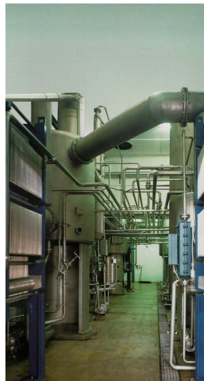
Installed Evaporation Plant
