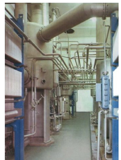
Installed Evaporation Plant
