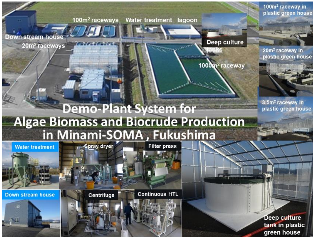
Figure 4: Demo-plant system for algae biomass and biocrude productions installed in Minamisoma city, Fukushima Prefecture. Photo by Watanabe, 2016
