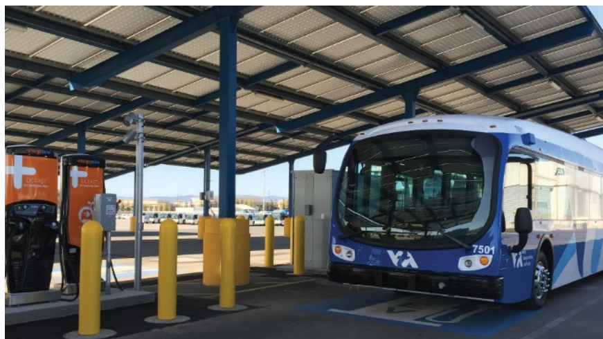
VTA is piloting a cutting-edge charging system designed to ensure minimal stress on California’s electric grid.
