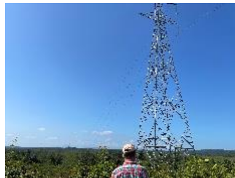
Photo 6 TRECESA transmission line "Río Frío" farm.
