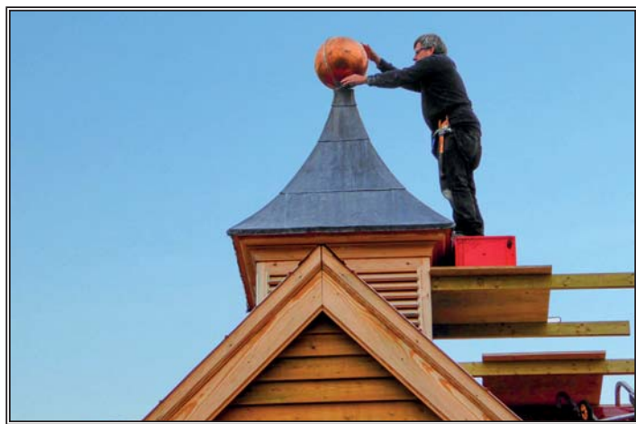
Master builder Phil Harris installs the crowning glory on our office. A 15" ball cock
