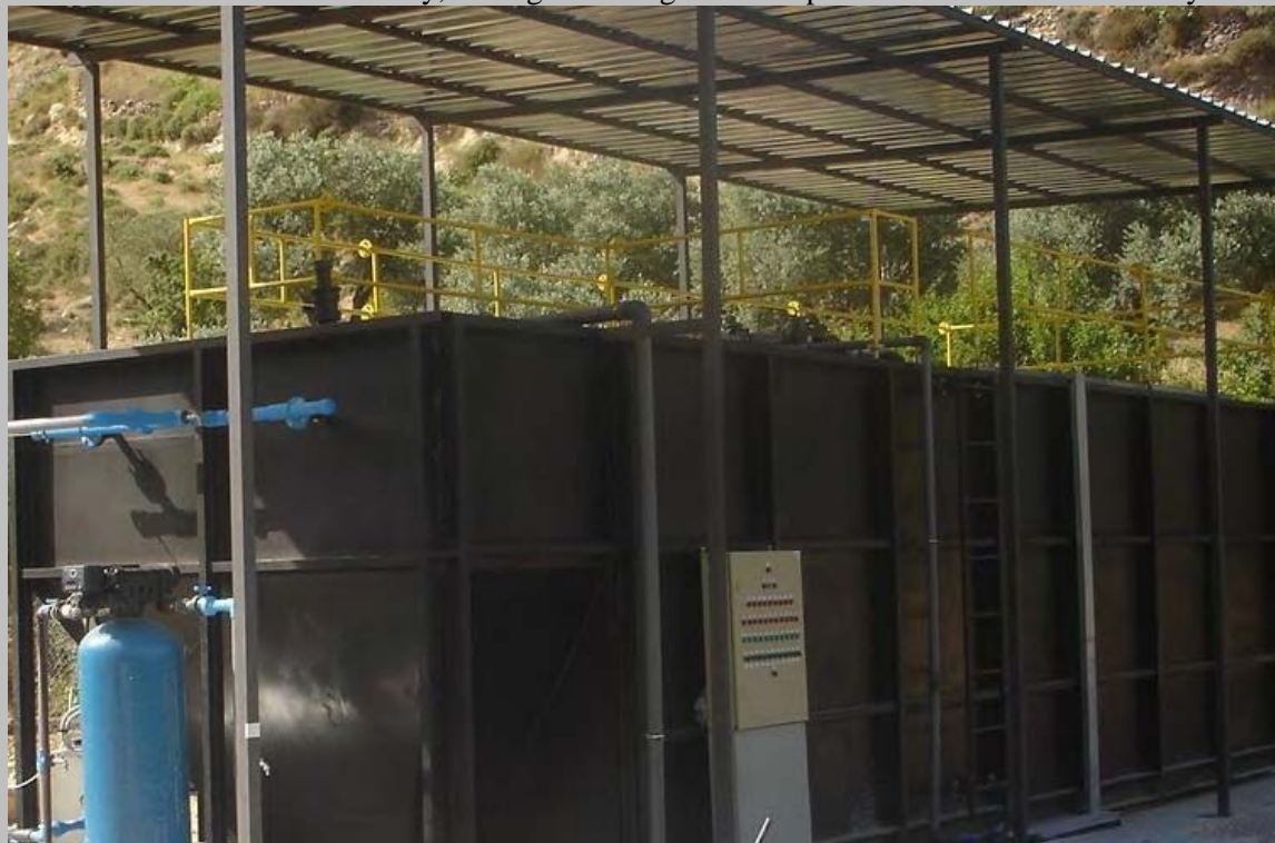
Photo 5.2.3: Nahaleen collective wastewater treatment plant – Bethlehem Governorate
