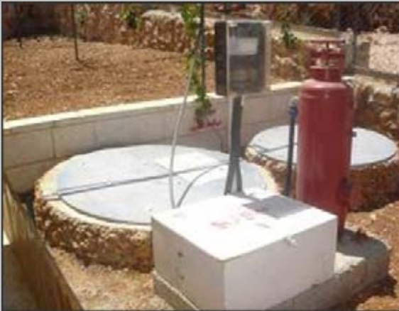
Photo 5.2.4: ARIJ's Small Scale Onsite wastewater Treatment Plants
