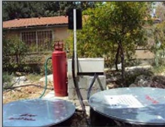
Photo 5.2.5: ARIJ's Small Scale Onsite Wastewater Treatment Plants
