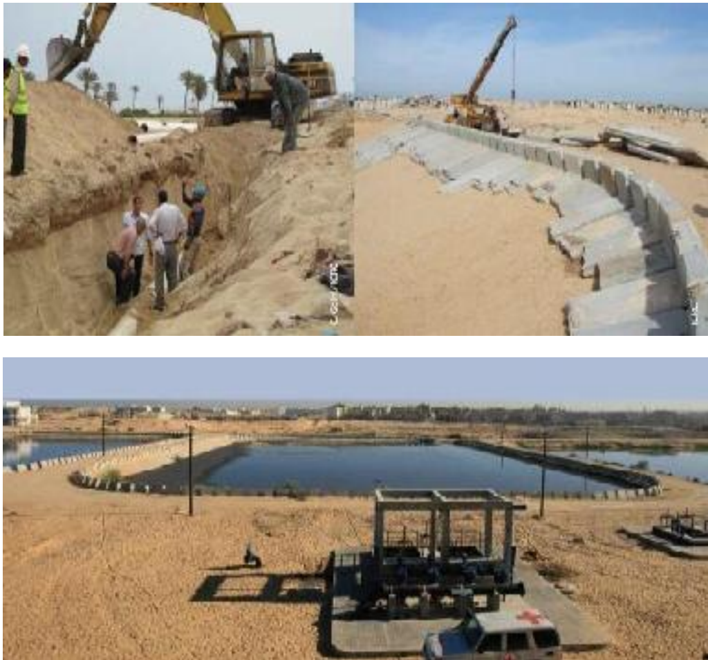
PHOTO 2.6: RAFAH WASTEWATER TREATMENT PLANT UNDER UPGRADE TO INCREASE ITS CAPACITY AND ENHANCE ITS EFFLUENT UTILIZING RECYCLED FRAGMENTS OF DEMOLISHED WALL SEPARATING GAZA AND EGYPT. (PHOTOS COURTESY OF ICRC)
