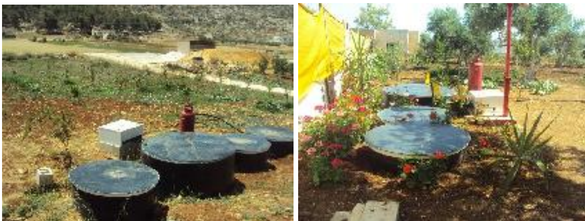
PHOTO 2.4: ARIJ'S SMALL SCALE ONSITE WASTEWATER TREATMENT PLANTS
