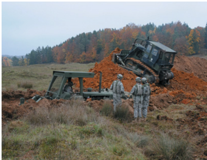
Engineers prepare defensive obstacles to defeat a conventional OPFOR attack at the JMRC. (DOD)
