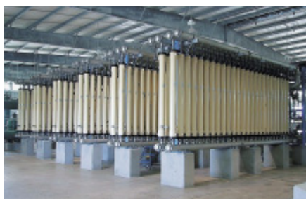
Microza™ modules at a water treatment facility
