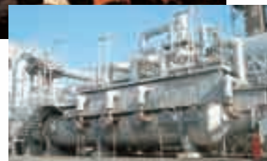
Equipment for thermal decomposition of the greenhouse gas N 2 O at the Leona Plastics & Materials Plant of Asahi Kasei Chemicals
