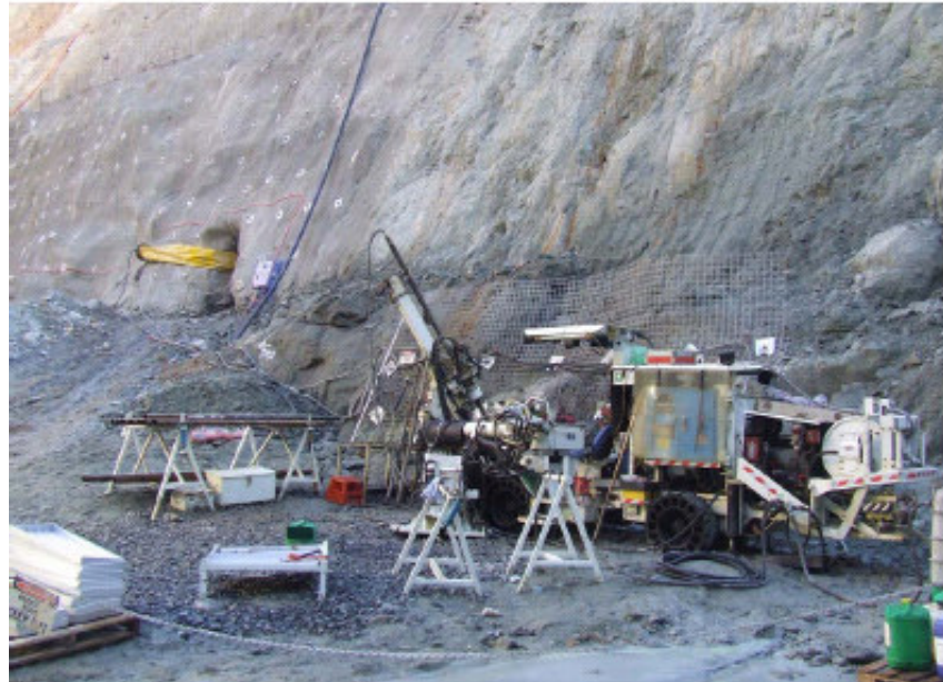
Diamond drilling in the base of Wattle Dam open pit with escape way portal in background
