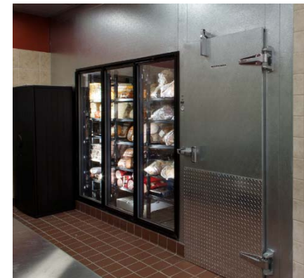
Food Storage/Walk-In Coolers
