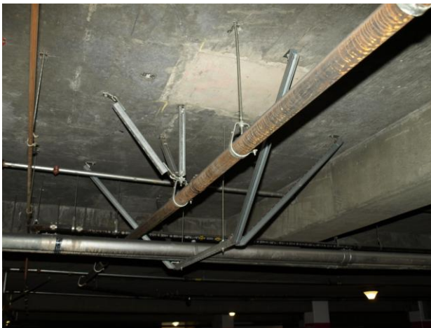
Figure MEP.3.1-6 Seismic Mitigation: Transverse bracing with J-hanger and strut at the restraining bolt. Note that longitudinal brace shown is ineffective because the J-hanger can slip along the length of the pipe.
