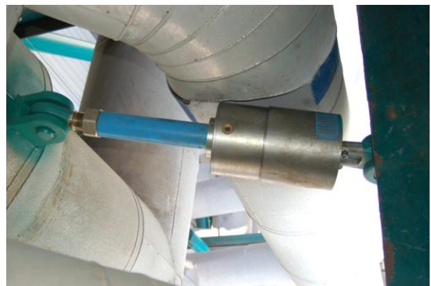
Figure MEP.3.1-6 Seismic Mitigation: Viscous damper used as restraint on large insulated pipe.
