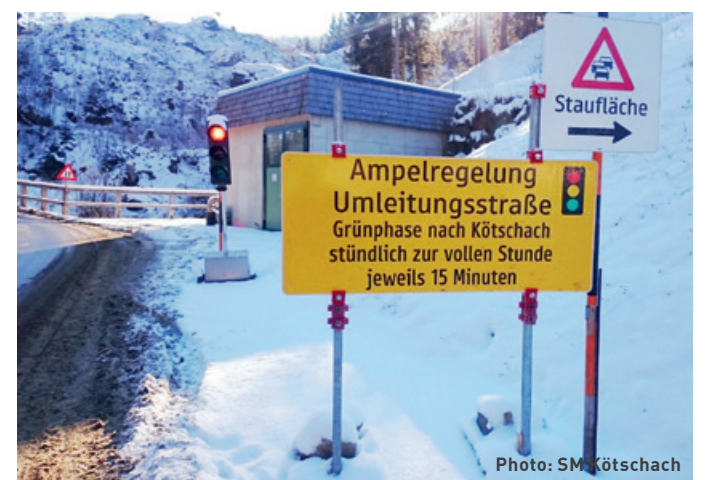
Traffic light control with MPB 1400 for the 4.6 km provisional bypass road. Announcement signs explain the fixed times for the green phase.
