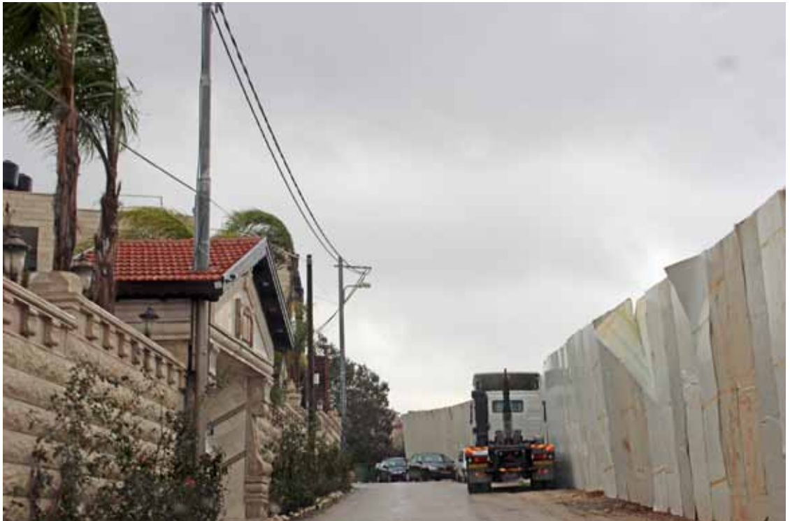
Construction work of Road Number 50 (Begin Highway) in Beit Safafa. February 2013 ©BADIL.
