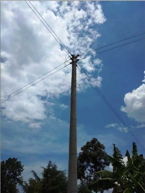
Low voltage single phase line and service cables in Kakamega and Nandi Counties
