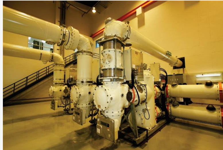
Gas Insulated Substation
