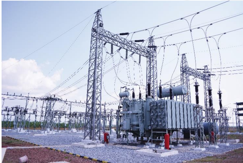
Air Insulated Substation
