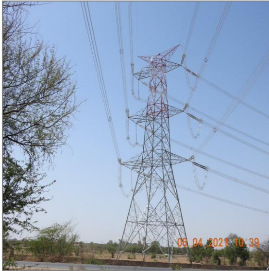
Phagi 765 kV D/C line along with associated bay for Rajasthan SEZ under Tariff Based Competitive Bidding (TBCB)
