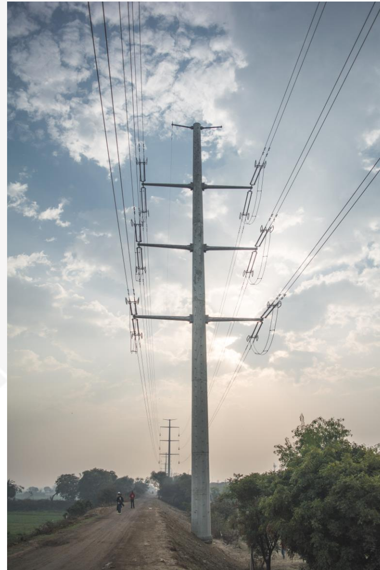
India's longest 400kV D/C transmission line with 94 Monopoles
