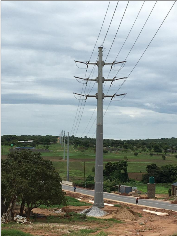
Construction of 132 kV Double Circuit Transmission Lines from Roma to Luska West
