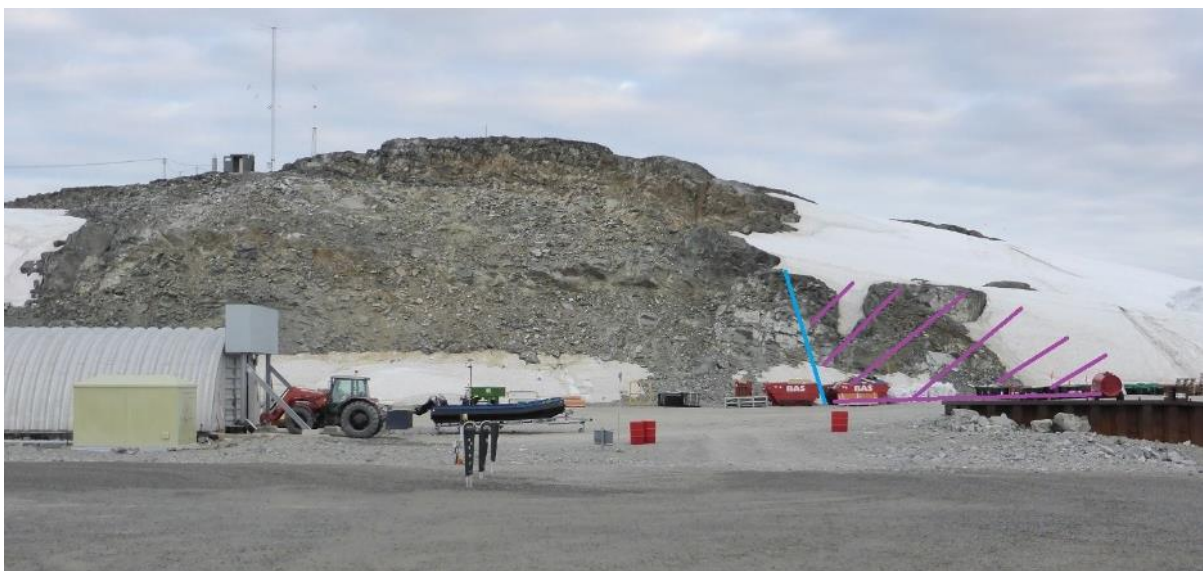
Figure 6 – Quarry stage one image from the west, showing the rock to be removed in purple hatching.
