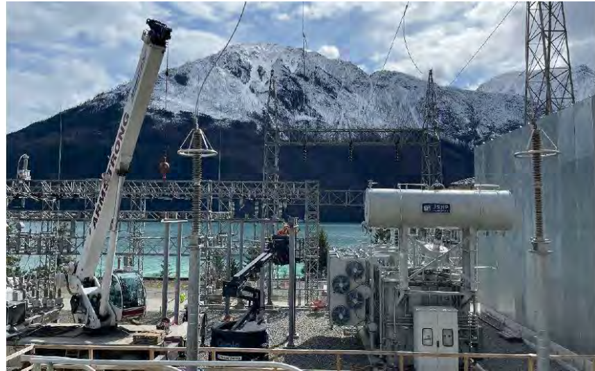
Above: In late March, crews worked to install steel components as part of the Transformer 3 replacement project at Bridge River 1. The project is expected to be completed this summer.
