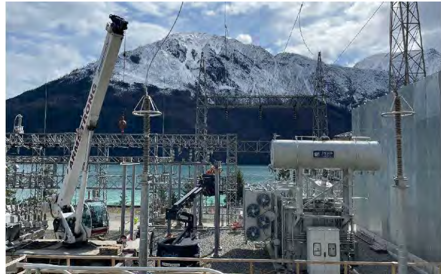
Above: In late March, crews worked to install steel components as part of the Transformer 3 replacement project at Bridge River 1. The project is expected to be completed this summer.
