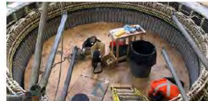
Crews have been busy with the pre-assembly work for units 7 and 8 at BR2.
