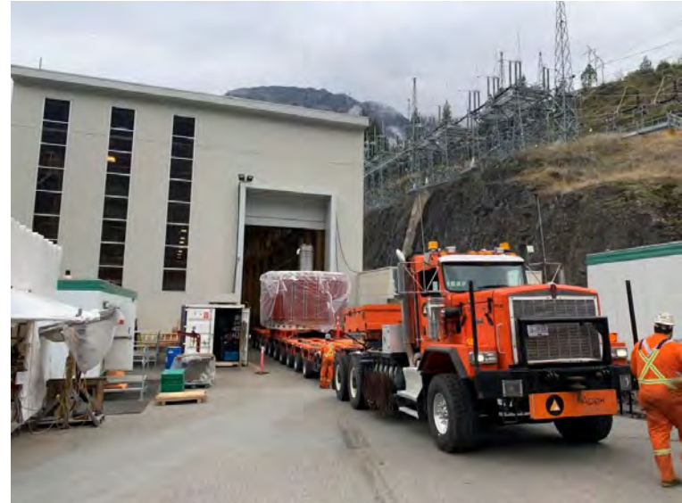
A newly assembled rotor is transferred from Bridge River 1 to Bridge River 2 for installation as part of the BR2 7&8 upgrade project.
