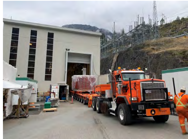
A newly assembled rotor is transferred from Bridge River 1 to Bridge River 2 for installation as part of the BR2 7&8 upgrade project.
