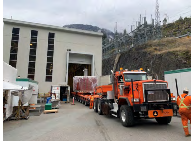
A newly assembled rotor is transferred from Bridge River 1 to Bridge River 2 for installation as part of the BR2 7&8 upgrade project.
