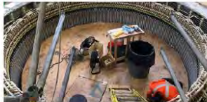
Crews have been busy with the pre-assembly work for units 7 and 8 at BR2.
