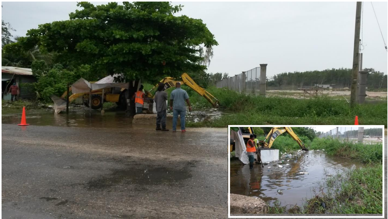
Figure 2.7e: MOW (Belize Office) clearing the clogged drain in front of Low’s Supermarket, Ladyville and to the left of the filled property (June 21, 2017).
