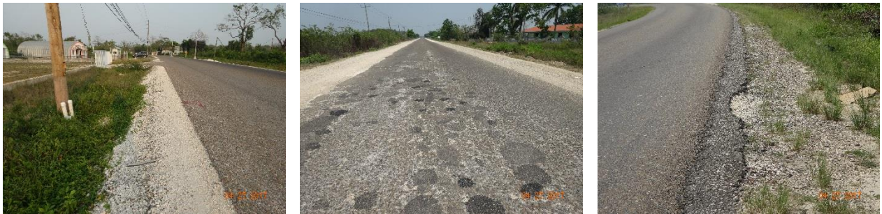
Figure 2.8: Pavement surface along Section 1. (Left) Recently surface-dressed pavement with paved shoulders (note no longitudinal side drains); (centre) Pavement in poor condition in the Lagos Community area; (right) Pavement surface in fair conditions with slight surface deformation and broken pavement edges.
