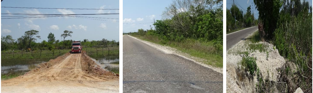
Figure 2.3: Longitudinal side drains are overgrown with vegetation and being filled up for new development between the junction of the old Northern Highway with the Philip Goldson Highway up to the Gardenia/Biscayne Village (mile 24.5).
