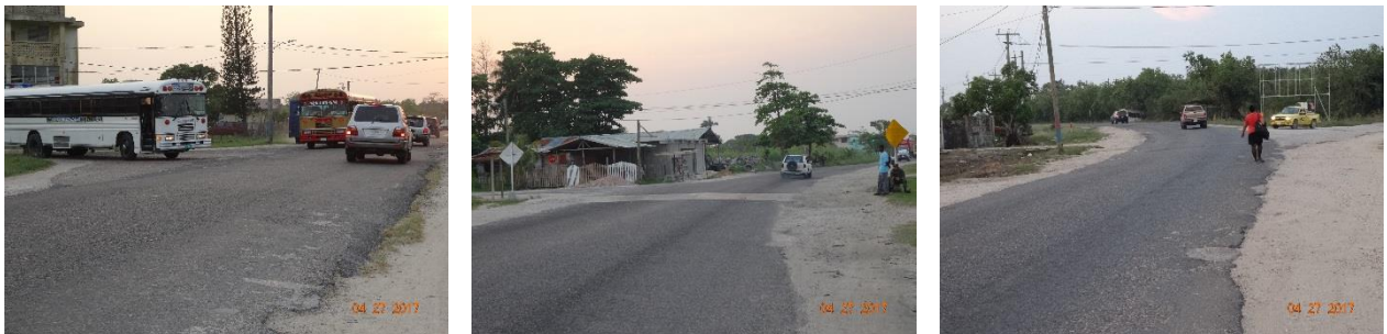
Figure 2.11: Price Barracks at mile 10 junction with the PGH. (Left) No traffic signs nor line markings to guide drivers; (Center) pedestrian crossing signs one is absent the other in dire need of maintenance; and (Right) pedestrian using the road carriageway as foot path.
