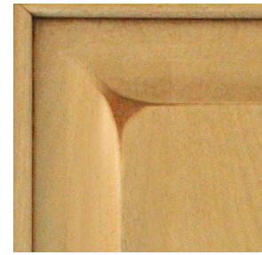
#4 - WORN CORNERS (ADD 5%) Profiles and corners are sanded down to remove the crisp new looking profiles.
