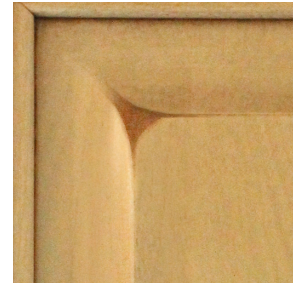
#4 - WORN CORNERS (ADD 5%) Profiles and corners are sanded down to remove the crisp new looking profiles.
