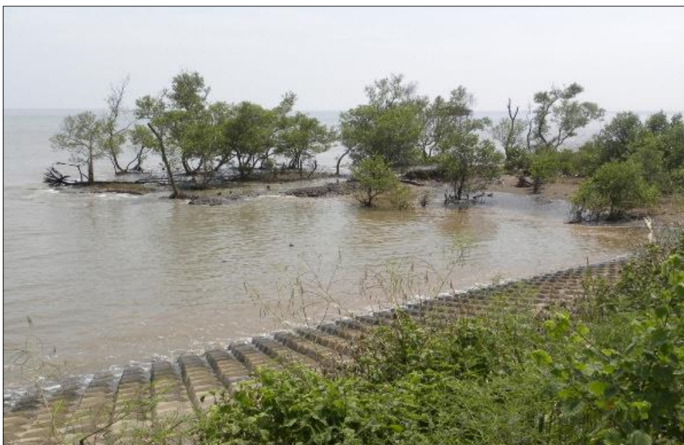
Figure 1. Coastal area in Vietnam with revetment on clay soil and remnant pocket of mangrove
