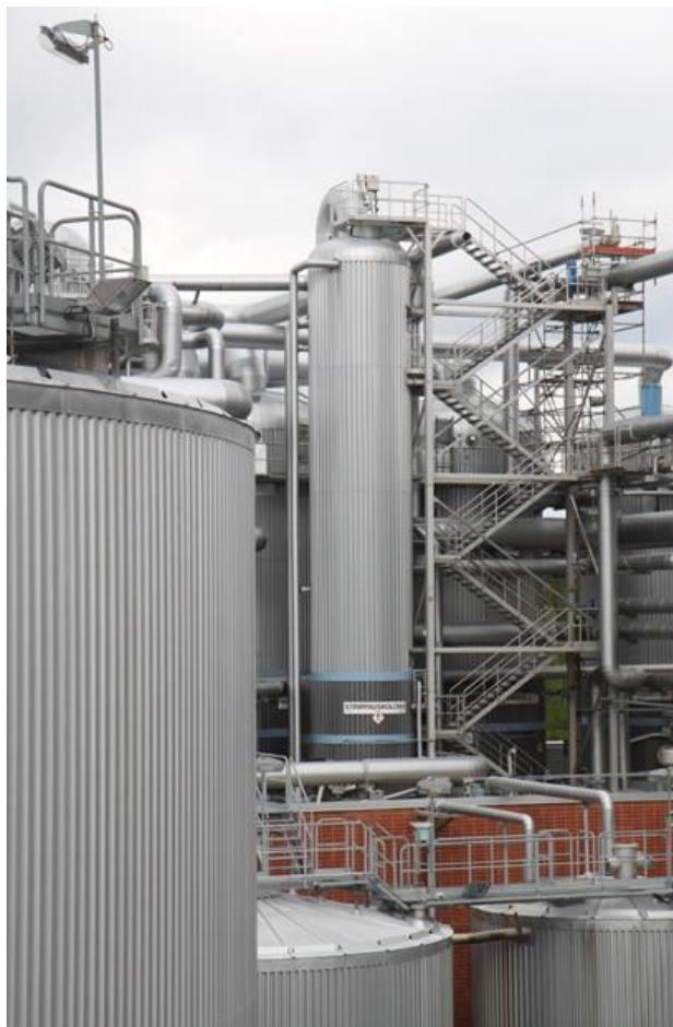
Figure 45: Separation of methanol from pulp mill: storage tanks and foul condensate stripping system (KnowPulp, 2019)
