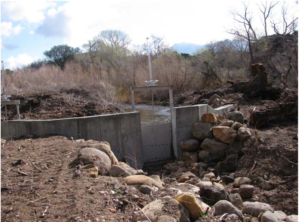
Figure 3. PacifiCorp Diversion on the Santa Clara River at Veyo © James McMahon
