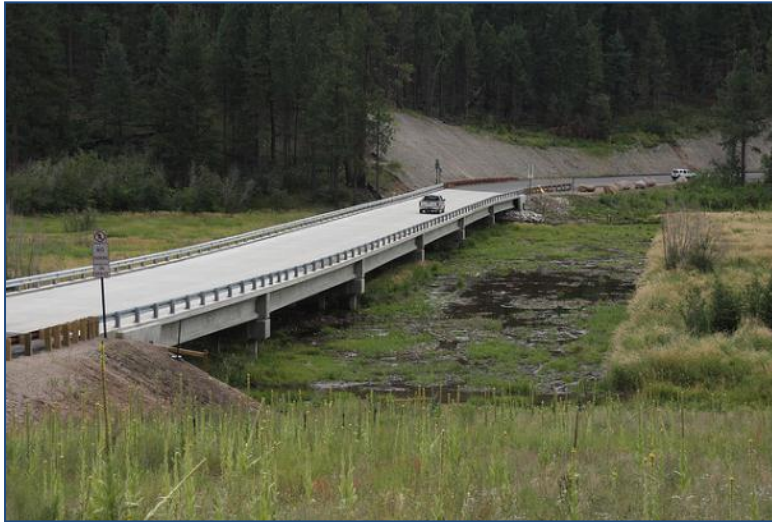
Figure 38. Construction of a new bridge on Highway 126, Jemez Mountains, New Mexico, in 2005 (photo courtesy of J.N. Stuart).
