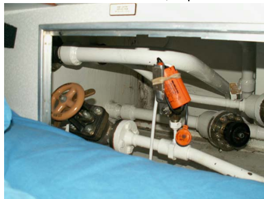
Figure 38: Valves located behind panel within cramped bunk space onboard a Trafalgar class submarine. Source: Author’s Image Archive
