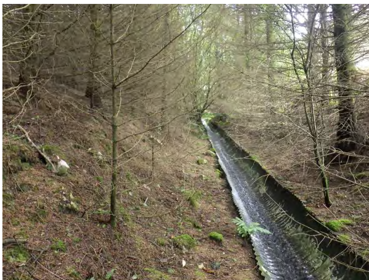
Plantation at TN4, showing the metal-lined ditch, with very little ground flora beneath the dense Sitka Spruce canopy.
