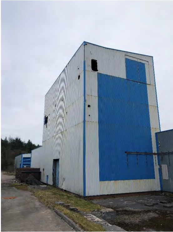
Photograph 3: Example of large opening on part of wall, on northern side of building A.
