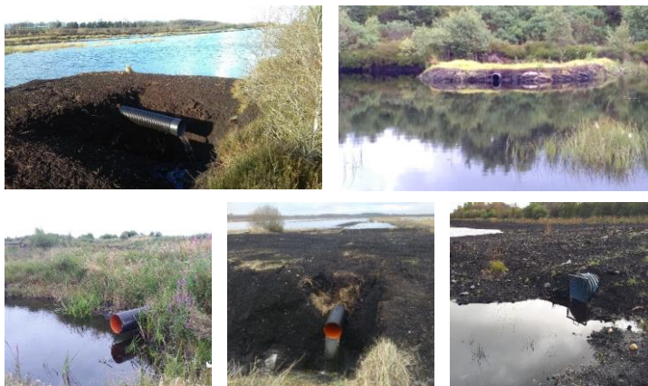
Plate 2-2: Examples of installed overflow pipes
