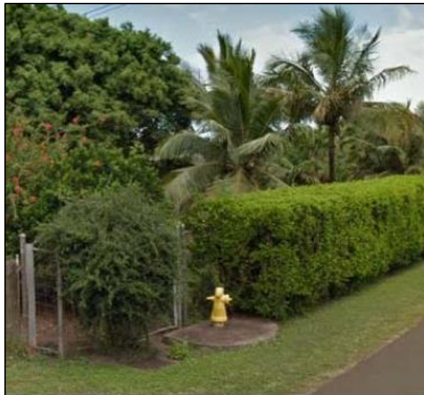
City fire hydrant that is more than one mile from nearest Mokulē'ia residence
