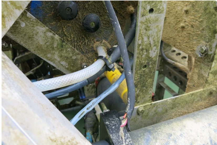
Figure 21 - The sheared cable that connected the Seaguard to the Hub
