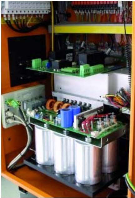
Figure 4: Switch cabinet with FischerLink
