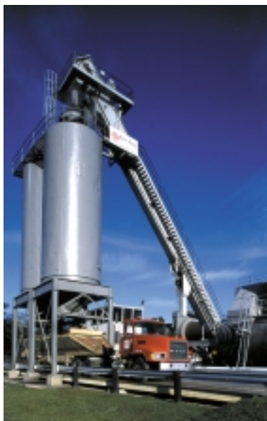
The Knox-Rivers plant near Augusta in the US.
