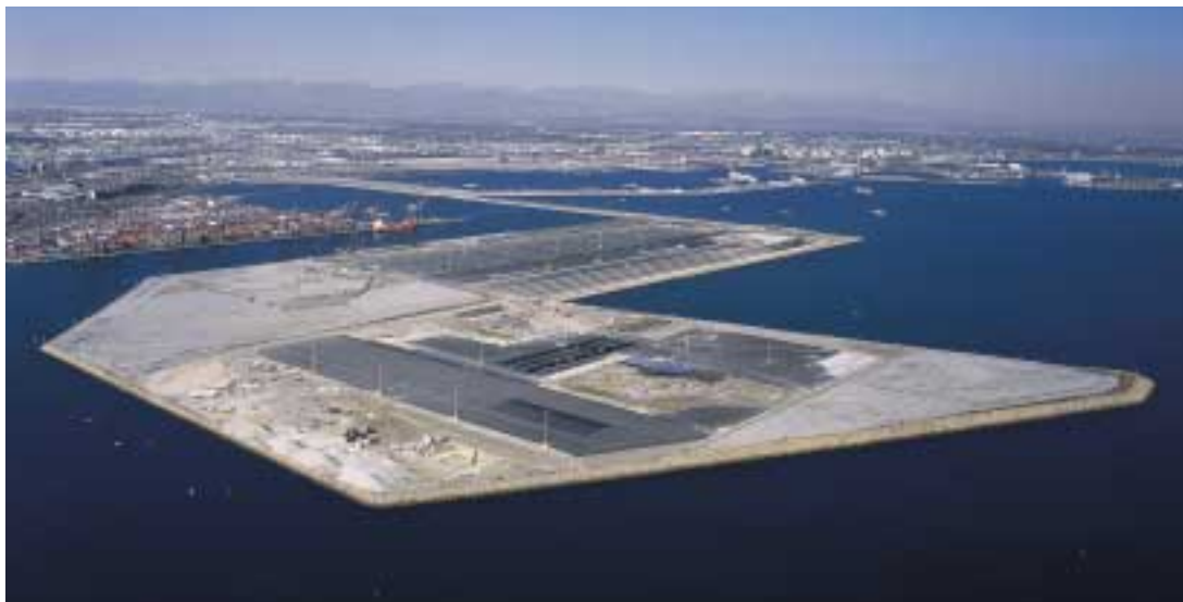
Construction of a 240-acre container storage and loading platform for the port of Los Angeles.
