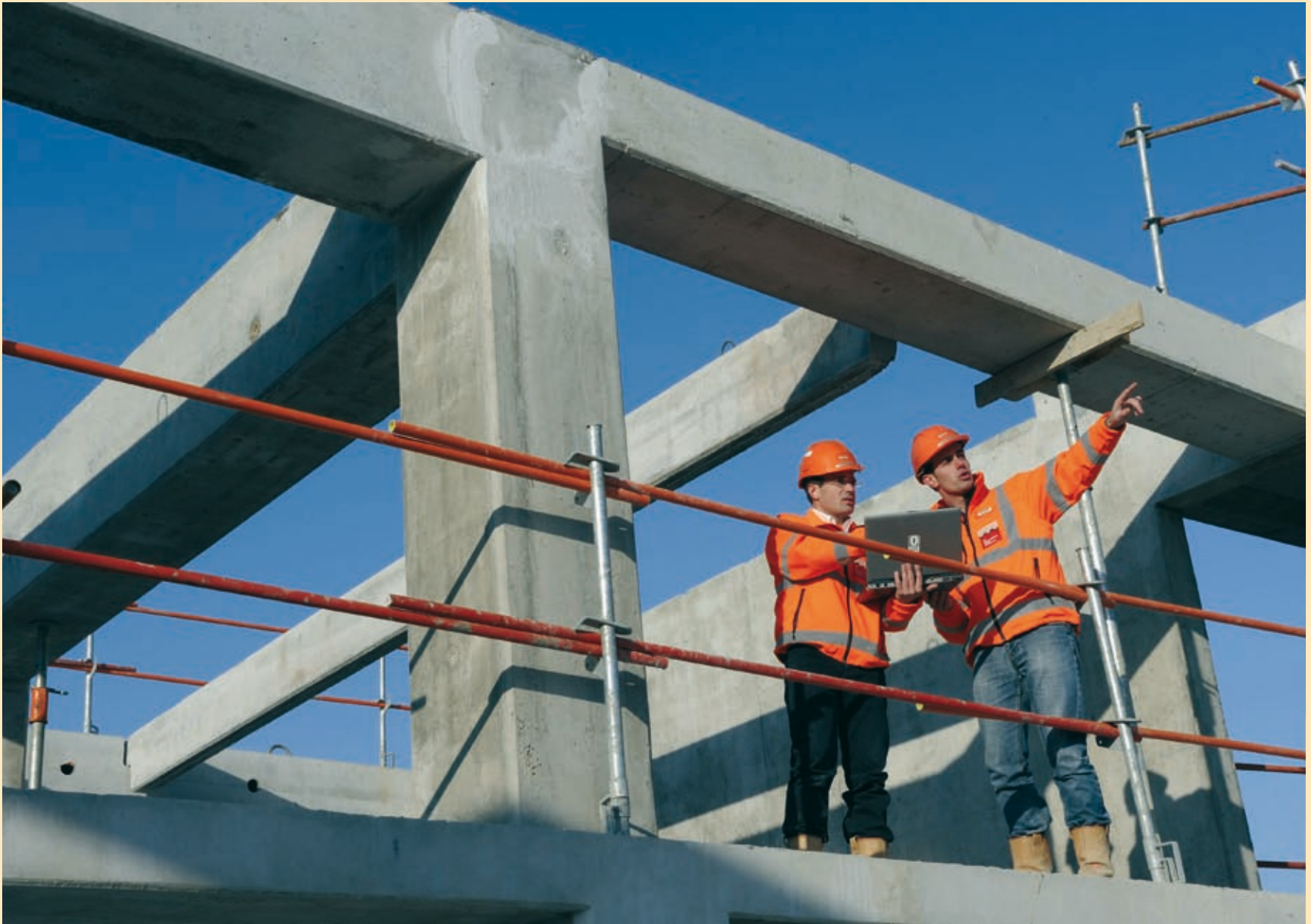
Nicolas Seailles and Jérôme Hollinger from Bouygues Bâtiment Ile-de-France on the site of the Aubervilliers shopping centre, near Paris
