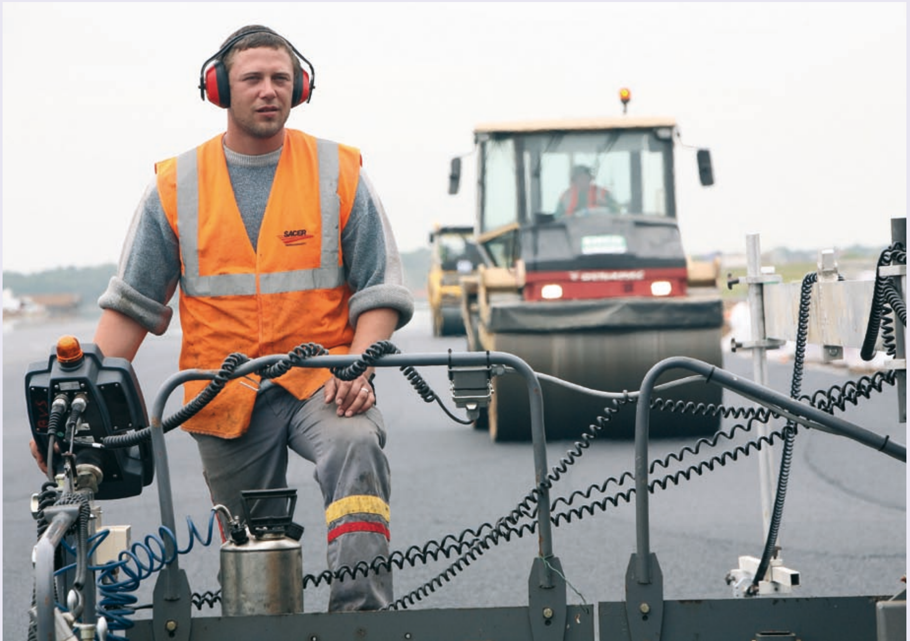
Jérémy Guerrin, an adjuster and finisher with Sacer PNE (Colas), at the Beauvais airport runway repairs site
