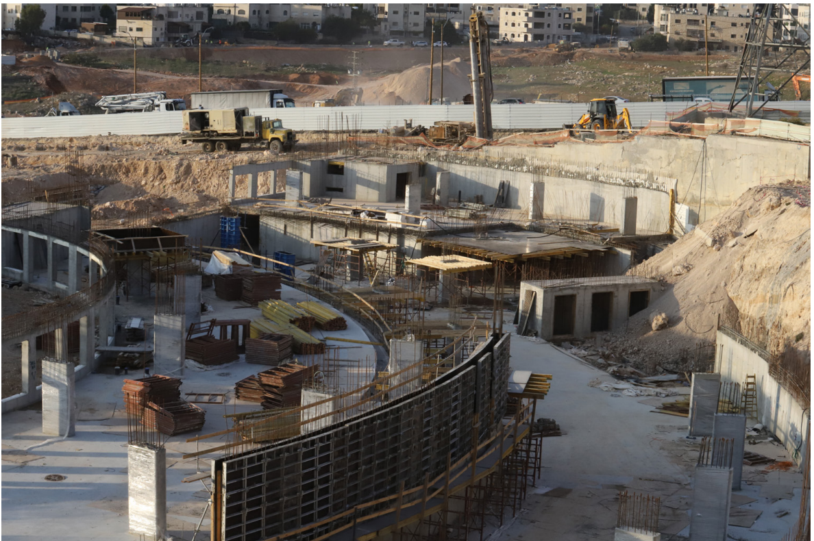
The "park and ride" lot under construction in the settlement of the French Hill
