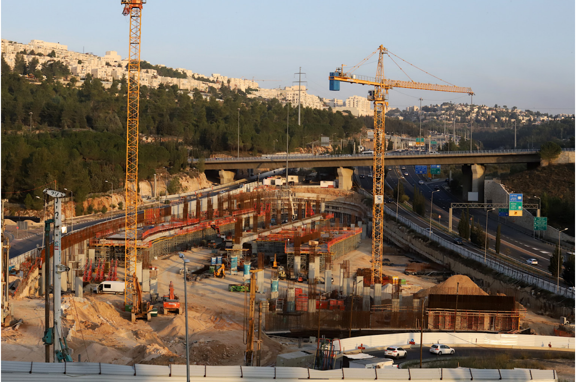
The "park and ride" lot under construction in the settlement of Ramot
