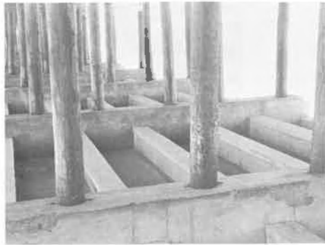
Fig. 15 The lowest point in the concrete is 2' above high water so that the concrete is never immersed in sea water which would otherwise cause spawling due to freezing and thawing. The timber piles are always exposed to complete wetting so that decay will not start due to the combination of creosote and salt preservation.
