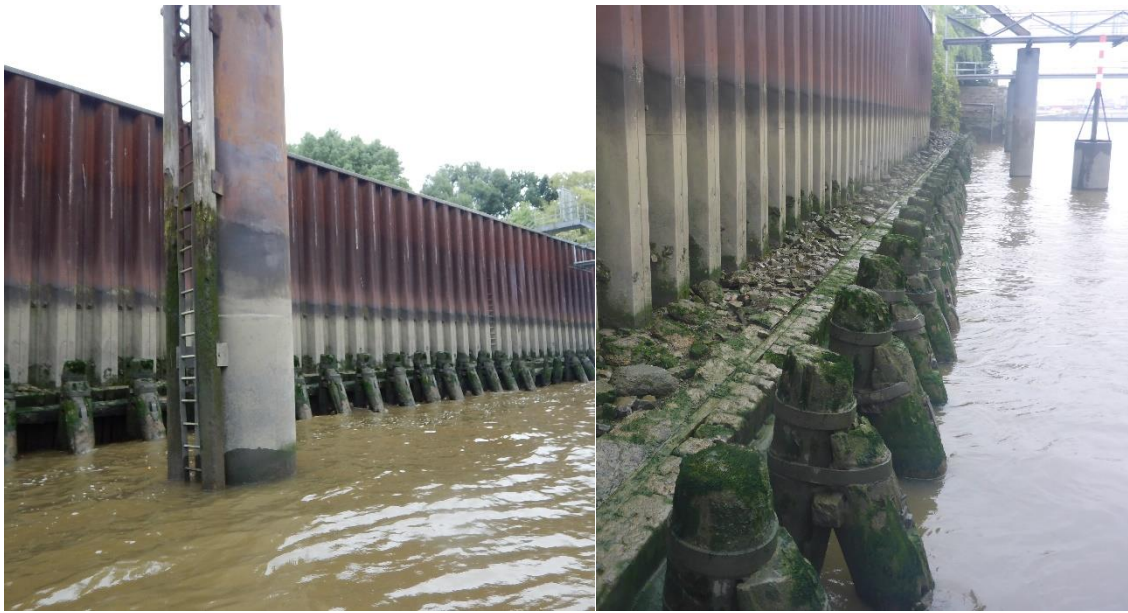
Figure 4: Metal pile mooring ( left ) and wooden jetty ( right ) at the “Petroleumhafen“ harbor site in the Port of Hamburg. (Image source: IfAÖ).
