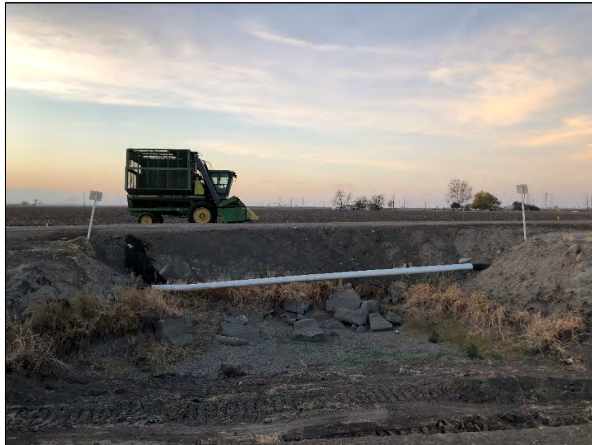
Figure 18: Exposed Gas Line, West Bank of Main Drain Canal
