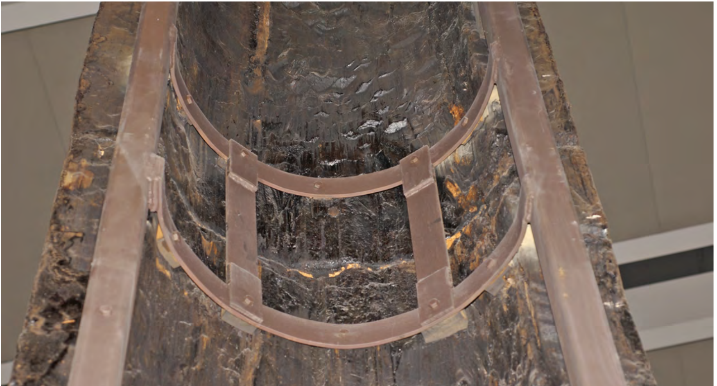
Figure 7b. Closeup of the horizontal metal straps with shims visible between the pole and the straps. Photo: Mylène Choquette, CCI (with permission from CMC).
