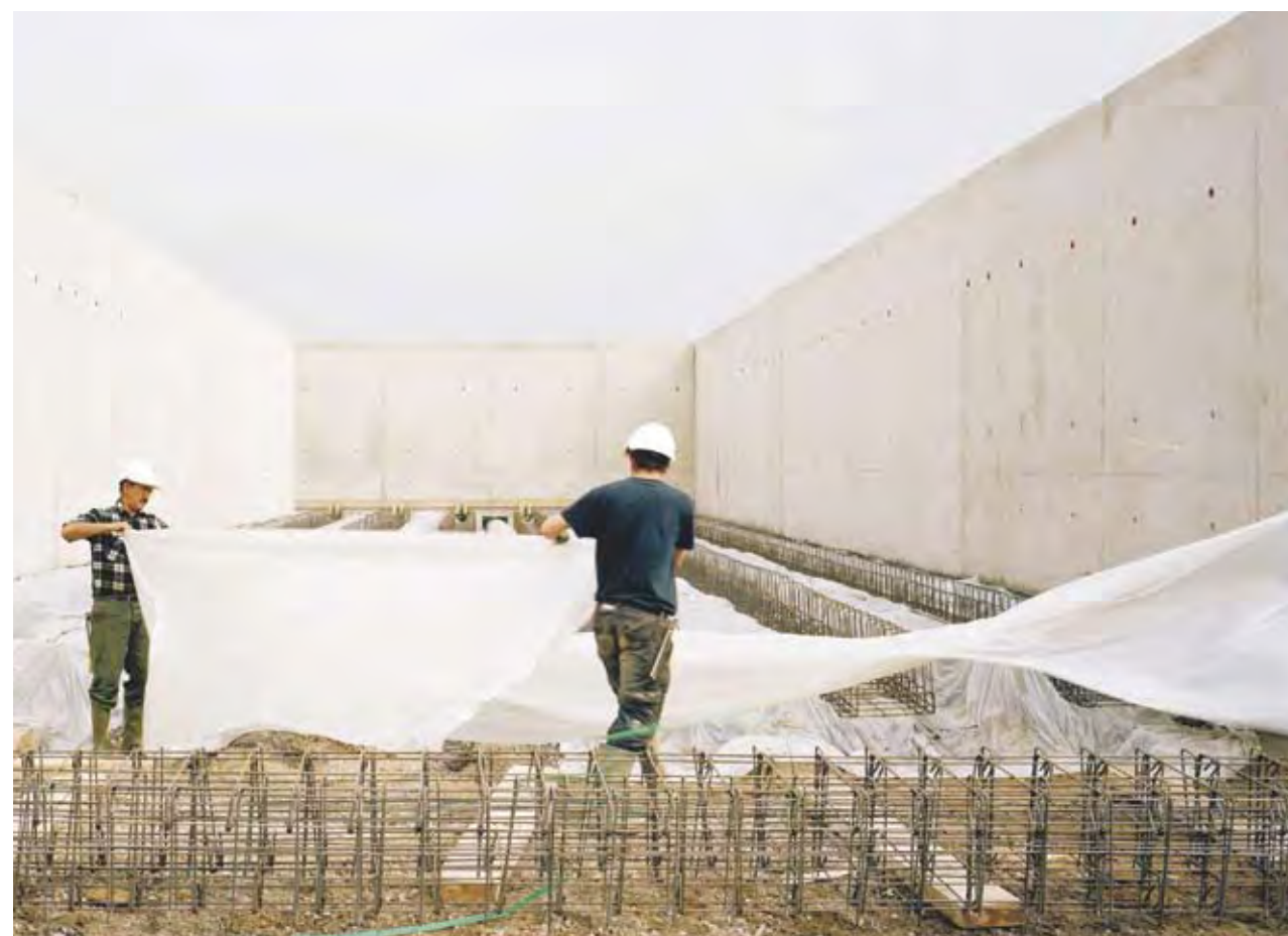
Work nears completion at the Ferti-NRJ methanisation plant at Passel (Oise). © JP Mesguen
