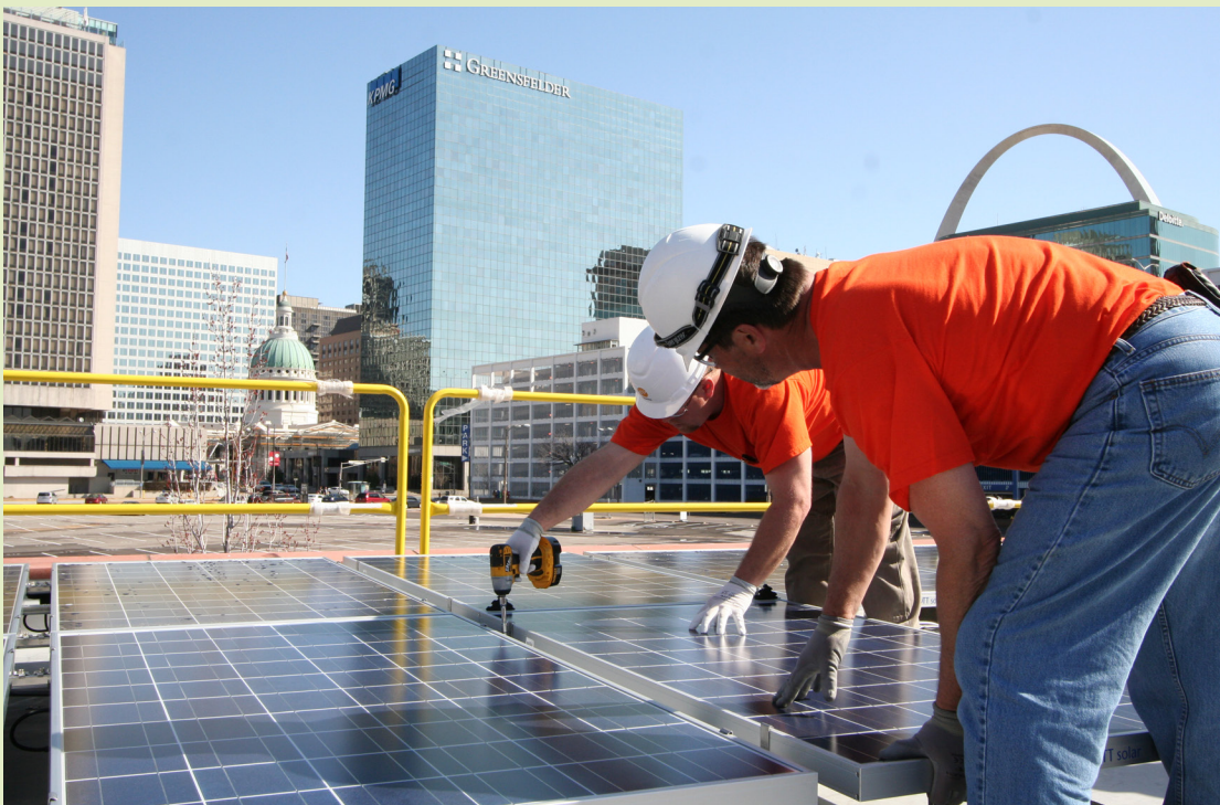
Busch Stadium solar installation by Microgrid Energy
