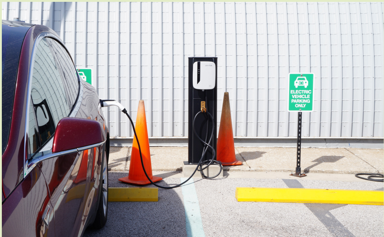
One of five EV charging stations at St. Louis Lambert International Airport
