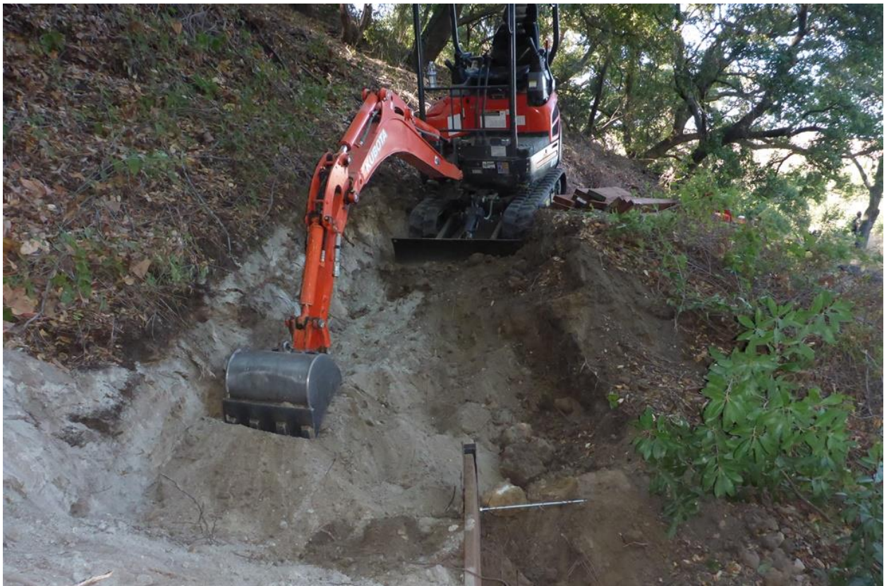
Narrow footprint excavator for excavation work on and near trails. Photo credit: Adam Maywhort.
