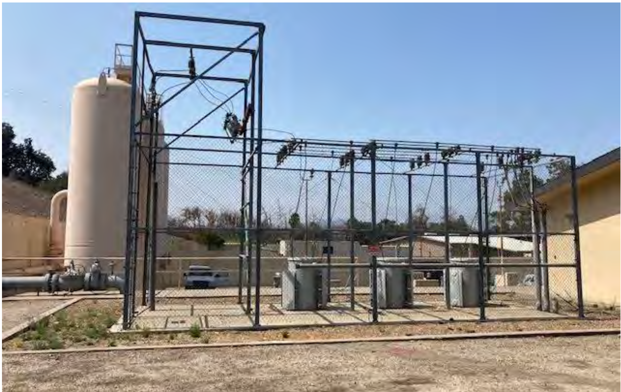
Figure 6 View of Electric Substation Equipment, View South
