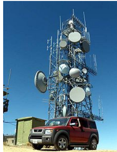
Figure 1 — Frazier Mountain in Southern California. Each dish provides a point-to-point connection with another location.
